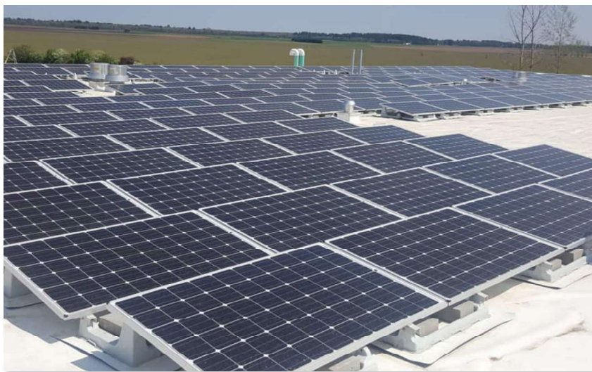
A good location for a solar project would be farmland or operating sites that will be with the business for years to come.
